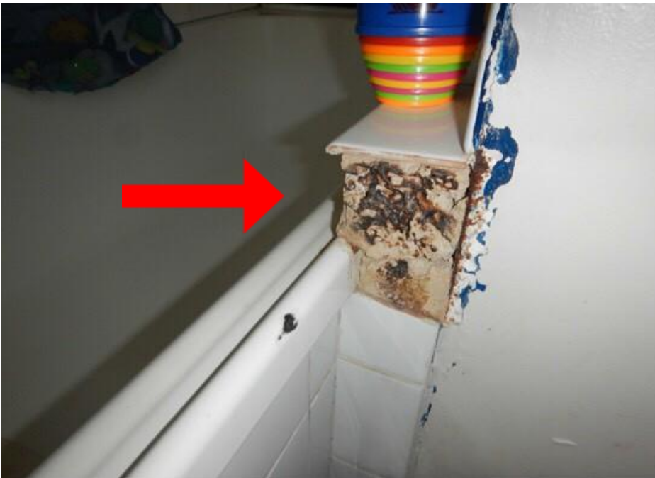
These photographs showed damaged areas in the bathroom.
