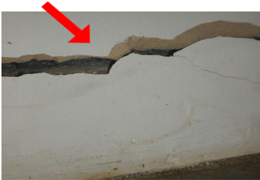
These photographs are of the fridge recess area, where cracking was most extensive.
